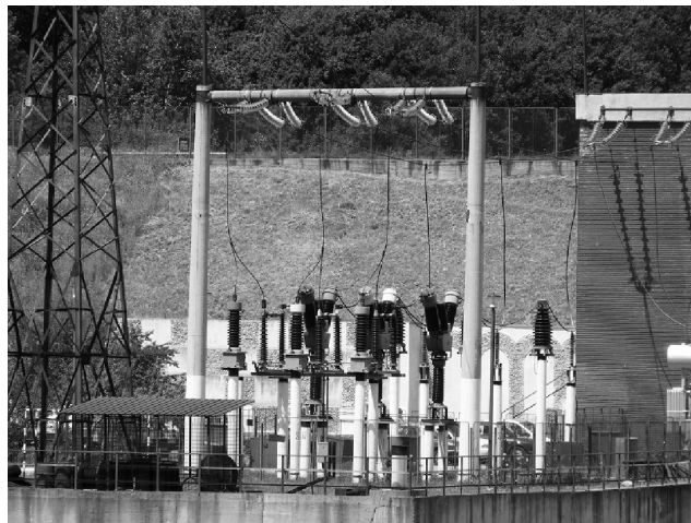
Figure 9.2 An electrical substation.
